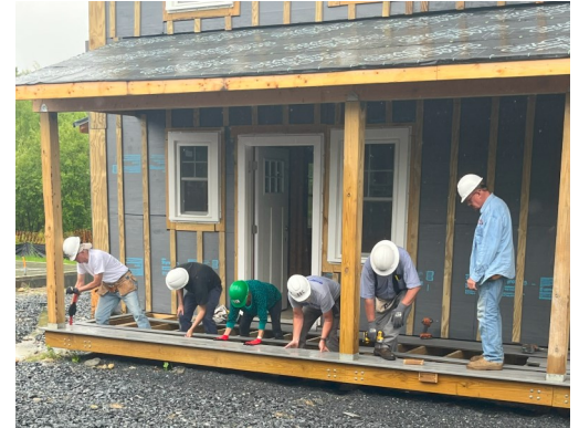
Part of the 2023 Missions Team working on one of the married couple housing duplexes.
